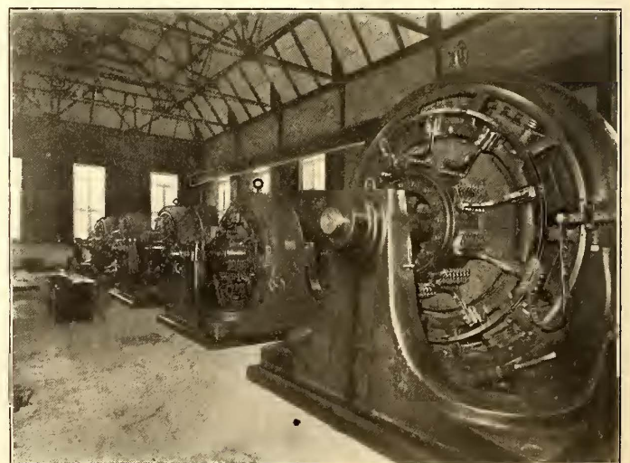
INTERIOR OF CONEY ISLAND SUB-STATION
