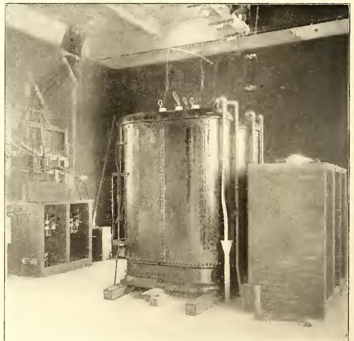
TRANSFORMERS IN SUB-STATION
