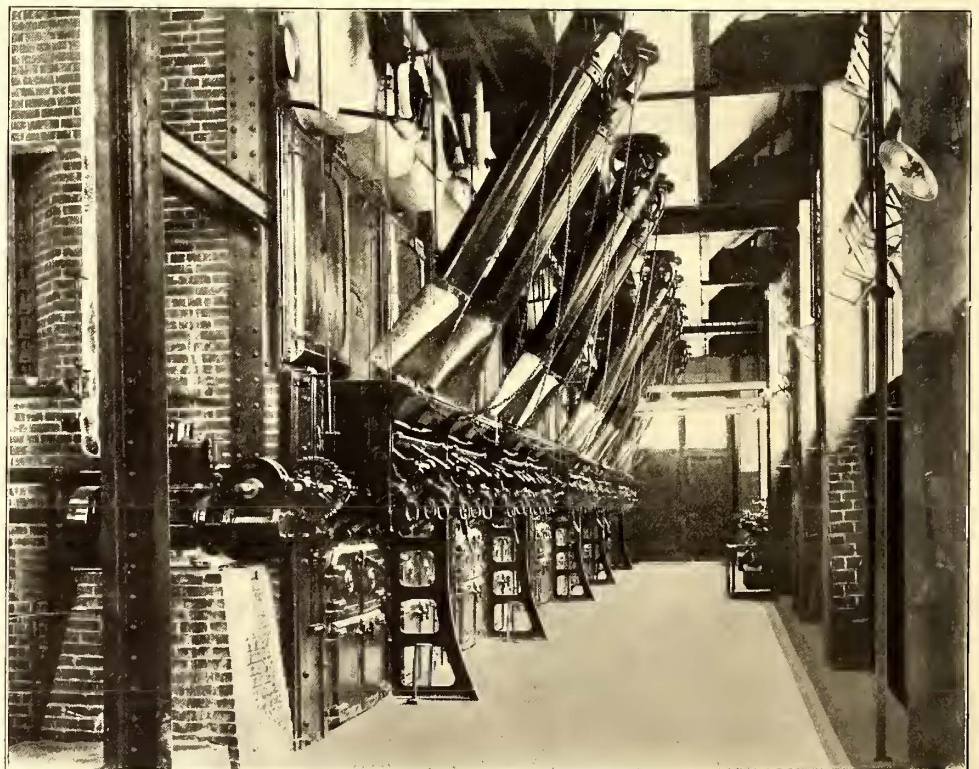
BOILER ROOM AND STOKERS
