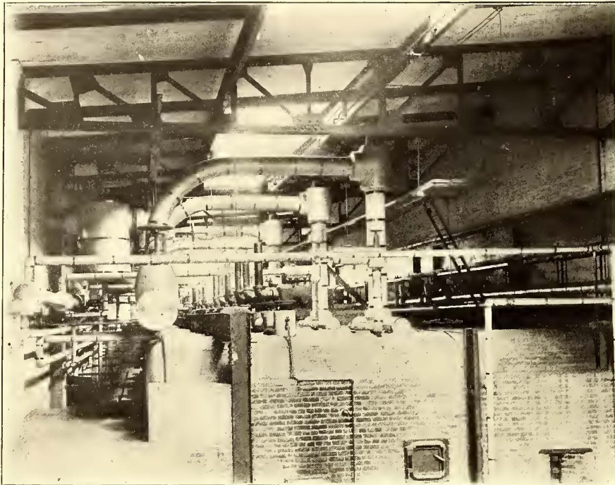
VIEW OF PIPING ABOVE BOILERS
