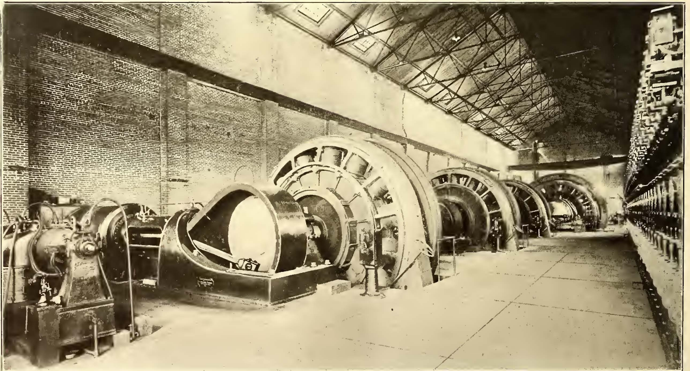
FIG. 9.—GENERAL VIEW OF ENGINE ROOM
