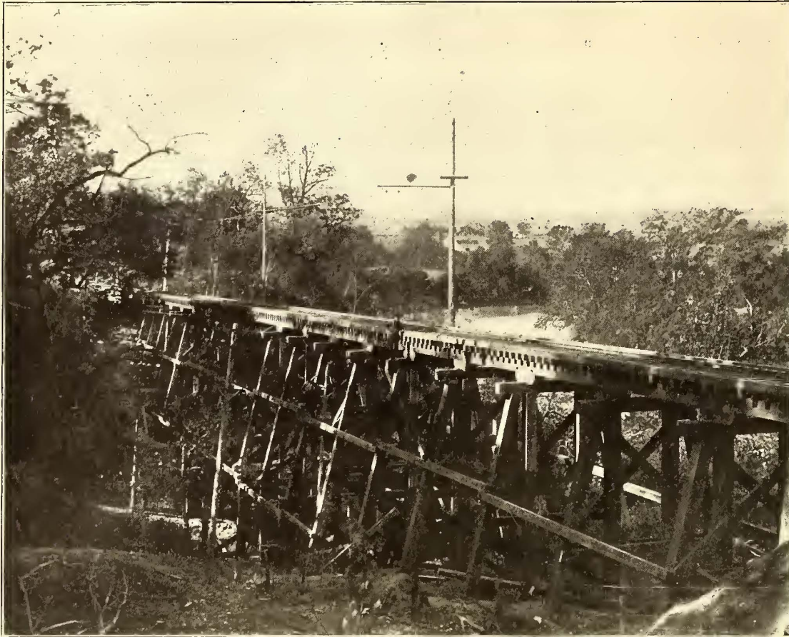
FRAMED TRESTLE 330 FT. LONG, CROSSING A RAVINE 60 FT. DEEP (RAPID DIVISION), NEAR KING'S MILLS
