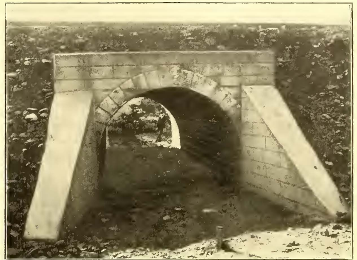
TYPE OF CONCRETE ARCH CULVERT MASONRY USED WHEREVER POSSIBLE IN CROSSING SMALL WATERWAYS
