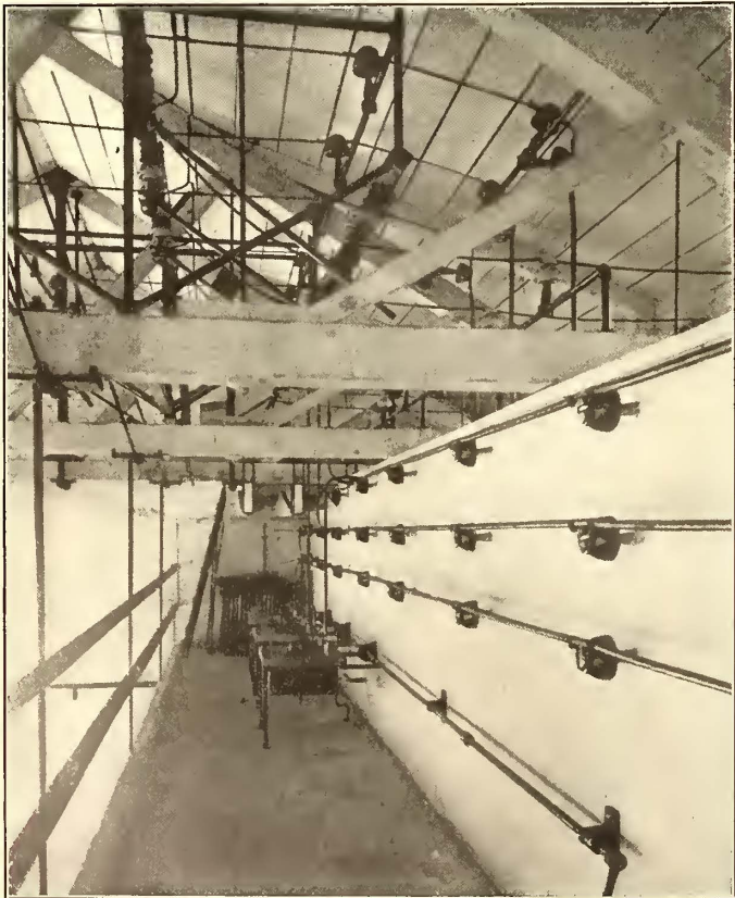
FIG. 10.—HIGH-TENSION GALLERY OF SUB-STATION, SHOWING HIGH-TENSION BUSSES, OIL SWITCHES AND HIGH-TENSION LINE SWITCHES
