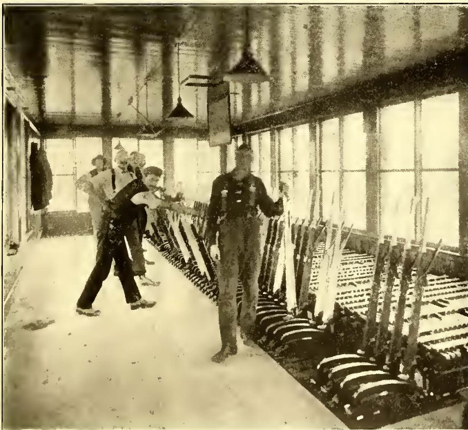
FIG. 7.—INTERIOR OF OPERATING ROOM OF CENTRAL SWITCH AND SIGNAL TOWER
