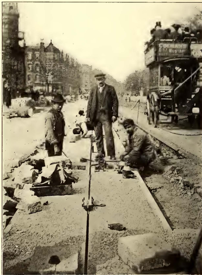
BONDING CONDUCTOR RAILS
