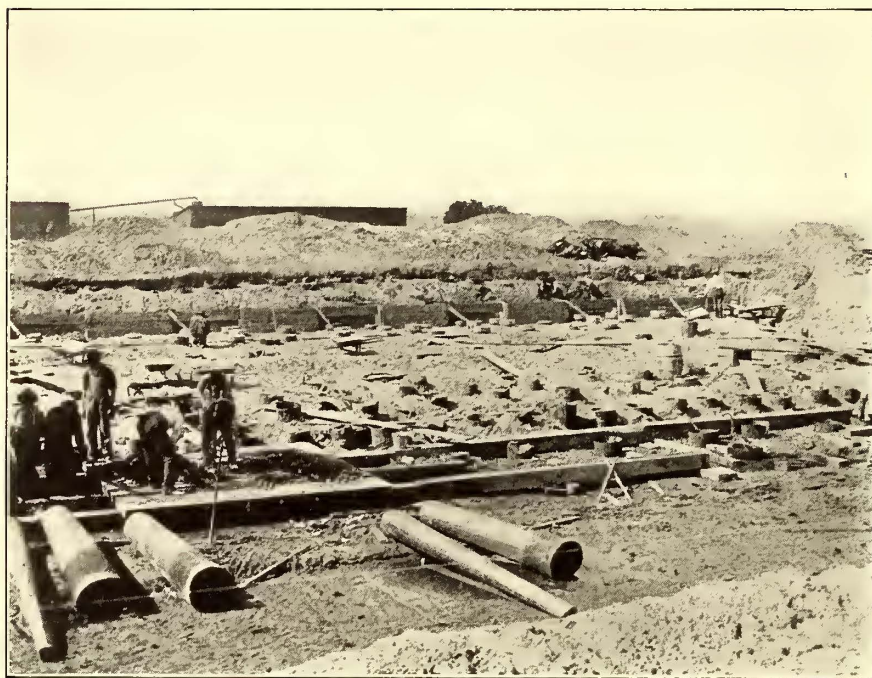
GENERAL VIEW OF THE DUBUQUE POWER PLANT FOUNDATIONS AFTER THE INSTALLATION OF THE RAYMOND CONCRETE PILES—SECTIONS OF THE SHEET-IRON SHELLS, USED IN DRIVING, APPEAR IN FOREGROUND
