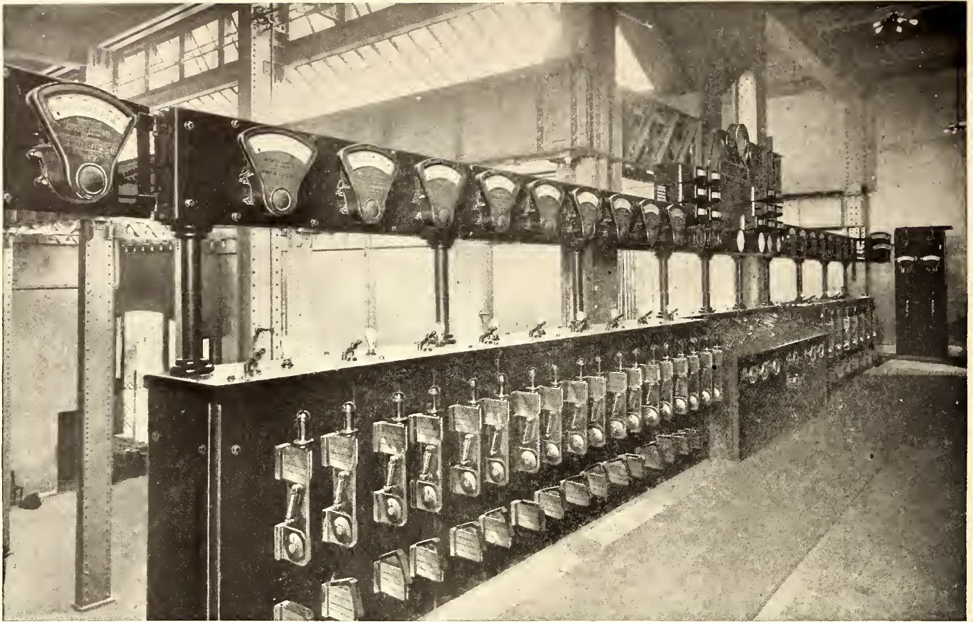
THE OPERATING SWITCHBOARD IN GALLERY—SUB-STATION NO. 11—SHOWING UNOBSTRUCTED VIEW ACROSS CONVERTER FLOOR BELOW
