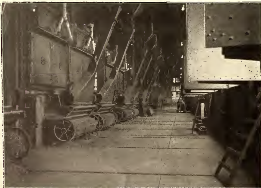
THE BOILER ROOM OF THE PARK AND VANDEVENTER POWER HOUSE OF THE ST. LOUIS TRANSIT COMPANY
