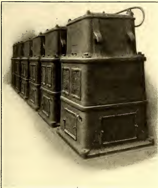
TWO GROUPS OF SUB-STATION STEP-DOWN TRANSFORMERS
