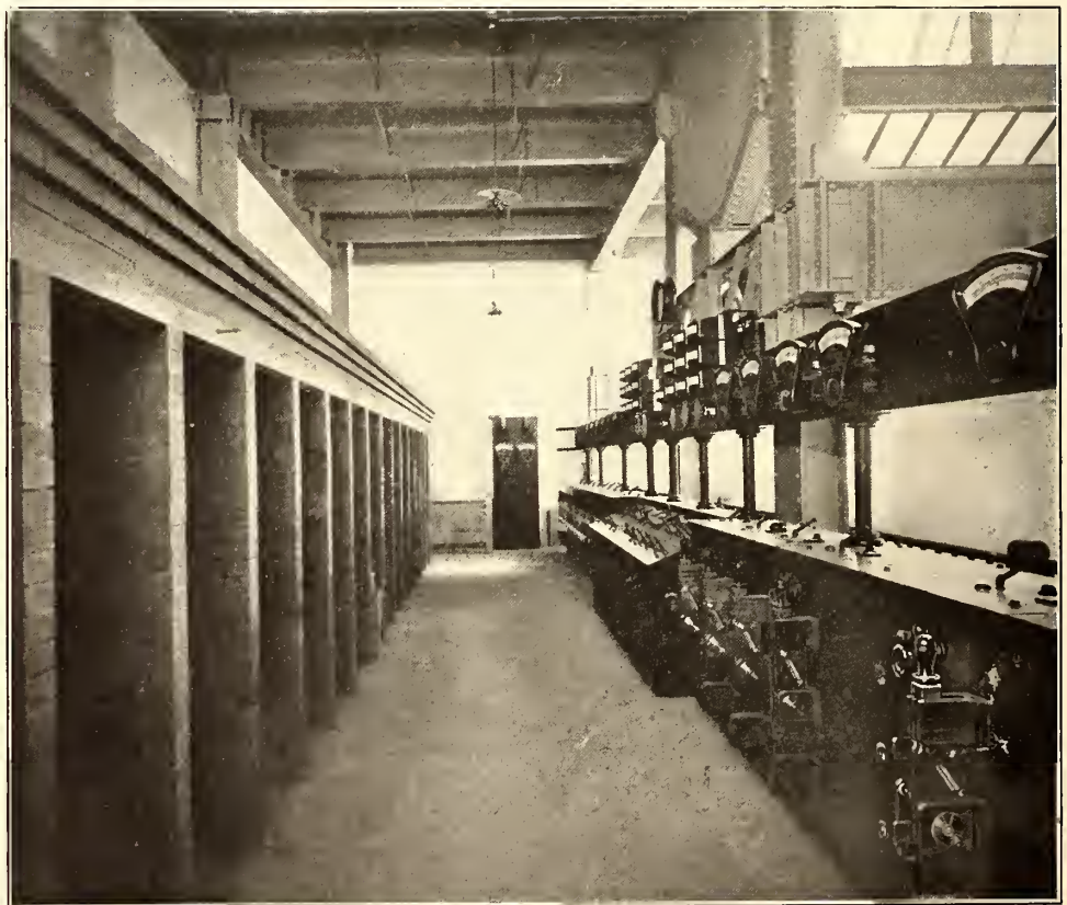
VIEW AT REAR OF OPERATING BOARD IN SWITCHBOARD GALLERY—SUB-STATION NO. 11—SHOWING COMPARTMENTS FOR THE DIRECT-CURRENT CIRCUIT BREAKERS
