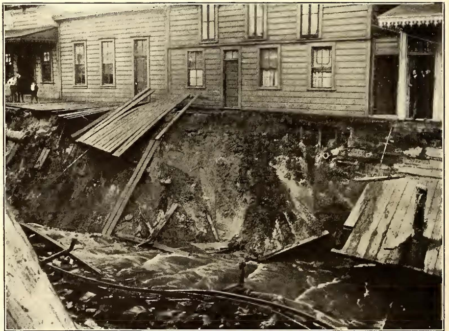
TRACK AT THE FOOT OF FILLMORE STREET, WASHED OUT FOR A DISTANCE OF 150 FT. THE TRACKS DROPPED 15 FT. IN ONE NIGHT
