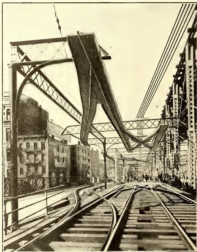
FIG. 1.—OVERHEAD CONSTRUCTION AT MANHATTAN TERMINAL, SHOWING OVERHEAD CONTACT BARS AND SHEET-STEEL TROUGHS.
