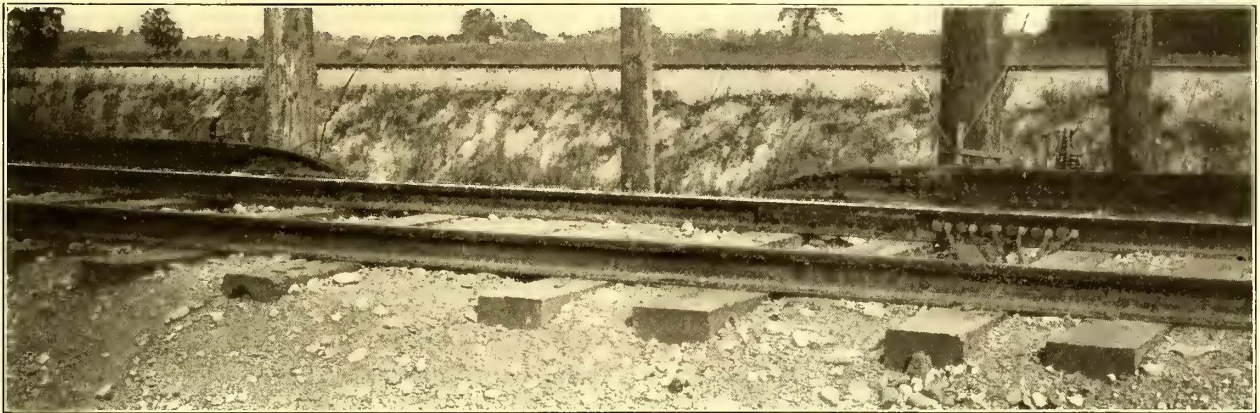
GROUND CONNECTION OF TRACK RAIL AT POWER HOUSE
