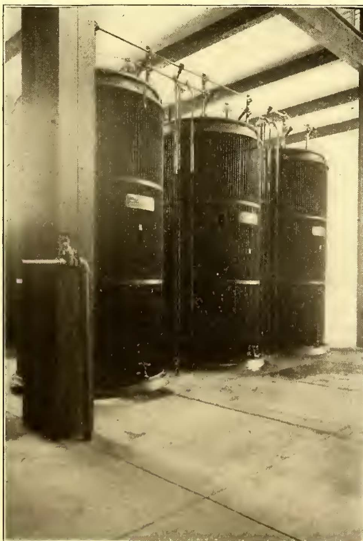
370-KW OIL-COOLED TRANSFORMERS IN MAIN POWER STATION
