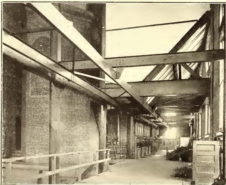
BOILER ROOM, SHOWING FUEL-HANDLING OUTFIT AND STOKERS
