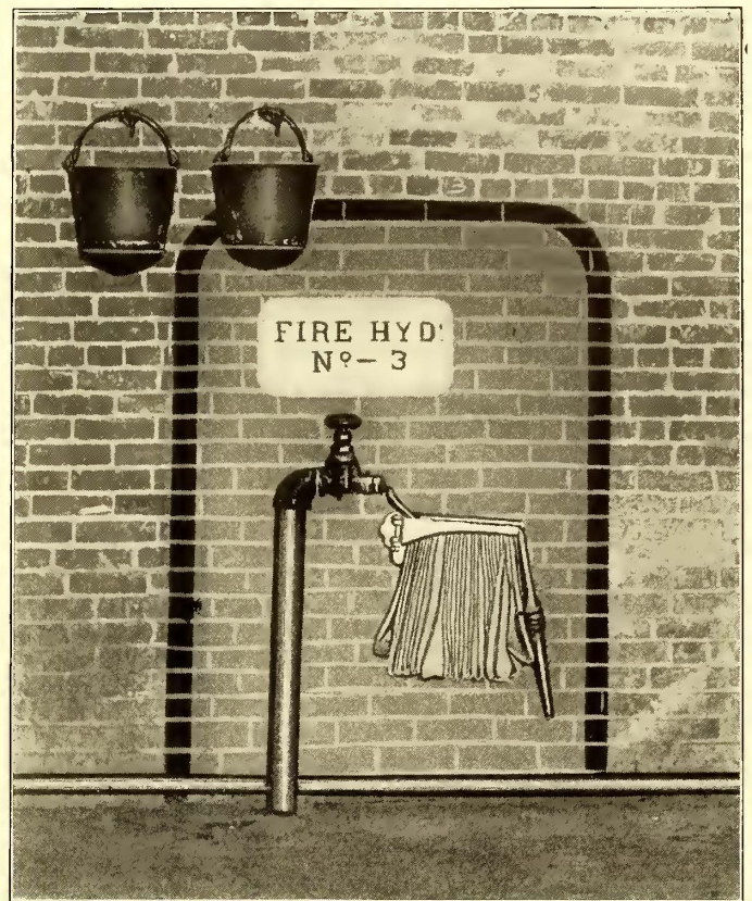
VIEW OF HYDRANT, ILLUSTRATING SCHEME OF PAINTING SPACE AT BACK OF HYDRANT
