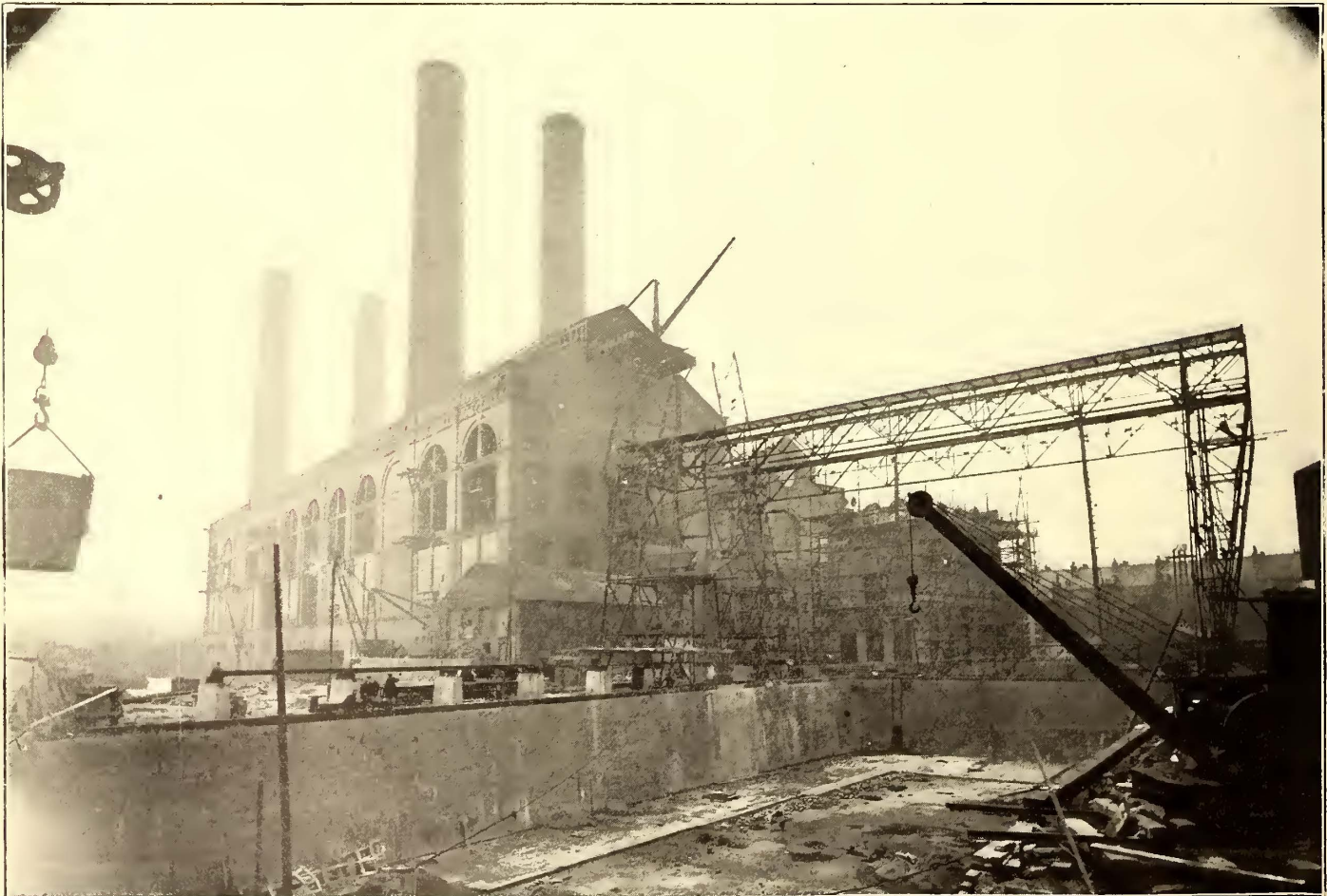
FIG. 17.—BARGE UNLOADERS AND COAL CONVEYORS AT CHELSEA GENERATING STATION
