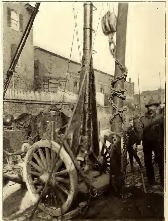
DERRICK WAGON IN ACTION, SHOWING ALSO CHAIN AND TACKLE AND THE USE OF CROWBARS TO LOOSEN THE CONCRETE AROUND THE POLE
