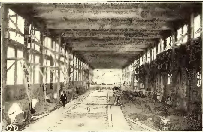
FIG. 6.—INTERIOR VIEW OF SHOP, SHOWING SCAFFOLDING FOR FILLING IN WINDOW SPACES. LAYING CONCRETE FLOOR TO PITS
