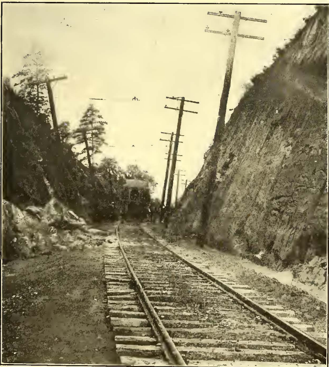
A CUT ON THE MAIN LINE, SHOWING TRACK CONSTRUCTION AND OVERHEAD WORK
