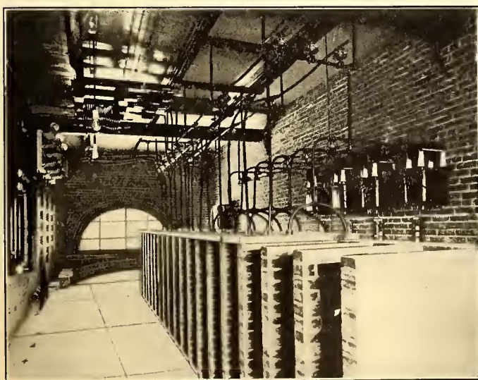
OIL SWITCH ROOM IN GALLERY OF BAY WINDOW
