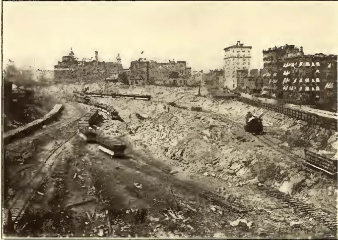
PART OF THE EXCAVATION FOR NEW GRAND CENTRAL STATION, LOOKING NORTH FROM FORTY-FIFTH STREET
