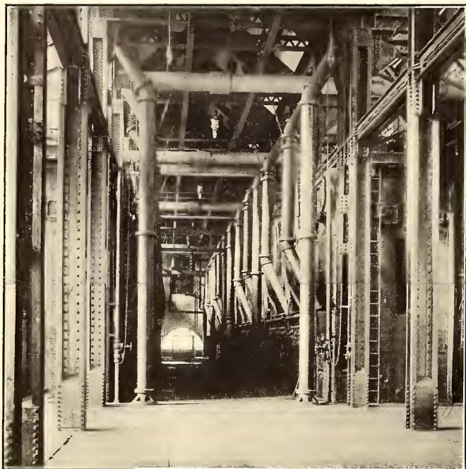
FIG. 6.—BOILER ROOM, SECOND FLOOR
