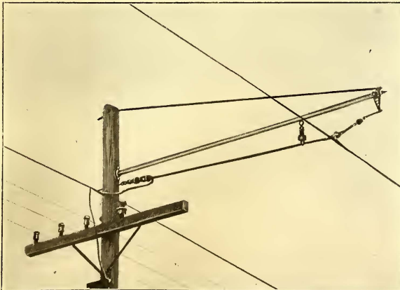
POLE TOP, SHOWING LIGHTNING ARRESTER TOP AND METHOD OF MAKING FEEDER TAP
