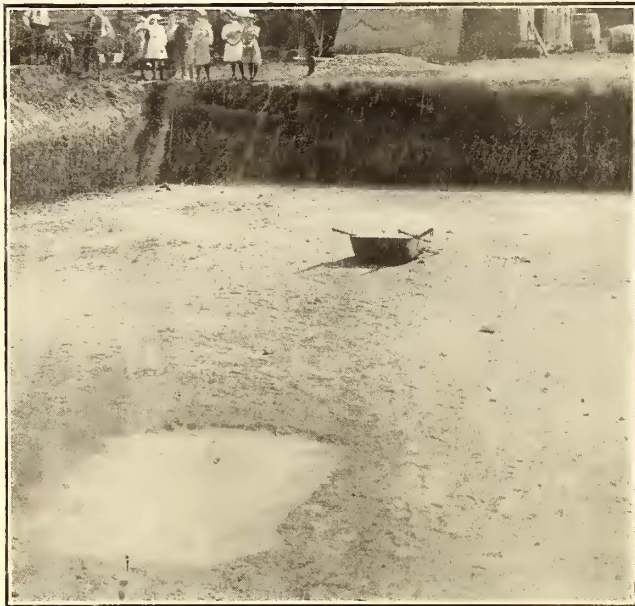
THE SENECA STREET EXCAVATION, WITH PORTION OF ROCK SWEEPED CLEAN TO SHOW ITS SMOOTHNESS
