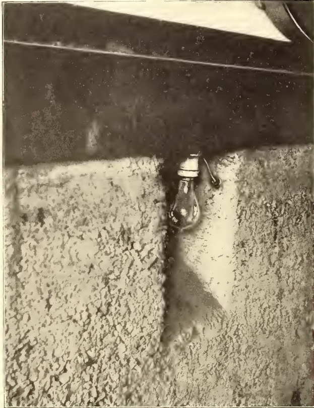
LAMP IN RECESS OF CONCRETE PIT
