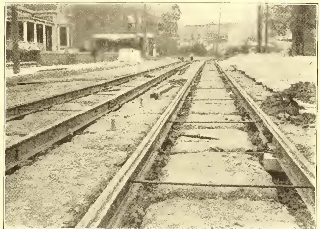
THE TRACK BEFORE CONCRETING, SHOWING THE METHOD OF SUPPORTING RAILS ON BLOCKS AND THE TWO SETS OF TIES
