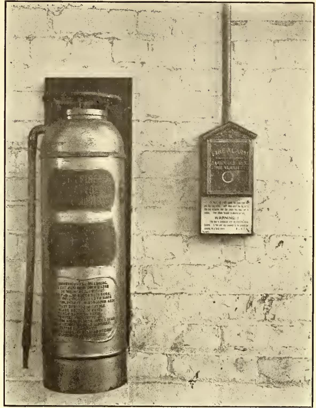
FIG. 7.—FIRE EXTINGUISHER AND INSIDE ALARM BOX
