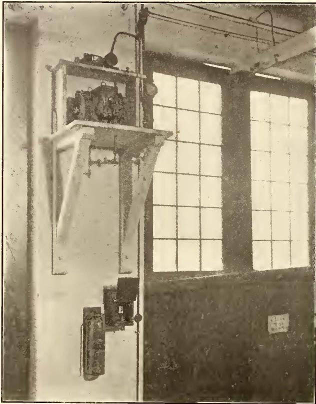
FIG. 16.—ONE OF THE COMPRESSOR MOTORS FOR THE SPRINKLER SYSTEM
