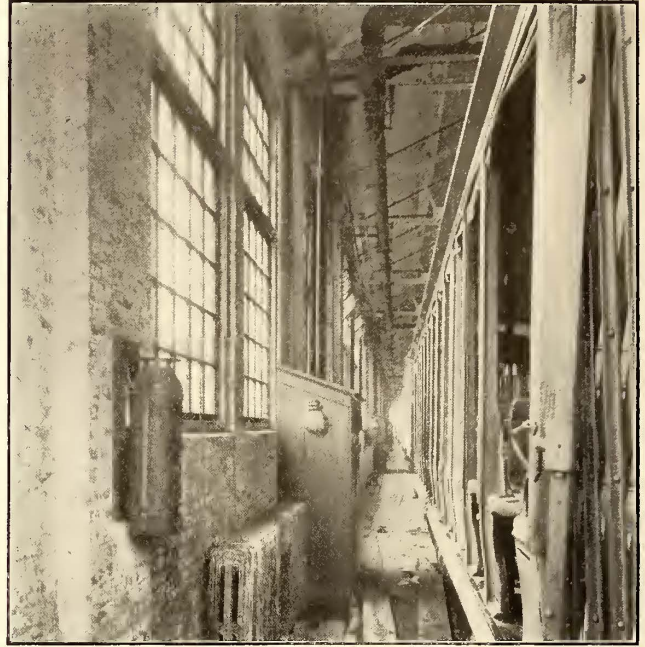
FIG. 5.—A VIEW ALONG AN AISLE, SHOWING A FIRE EXTINGUISHER, DRY VALVE BOXES, GONGS, ETC.
