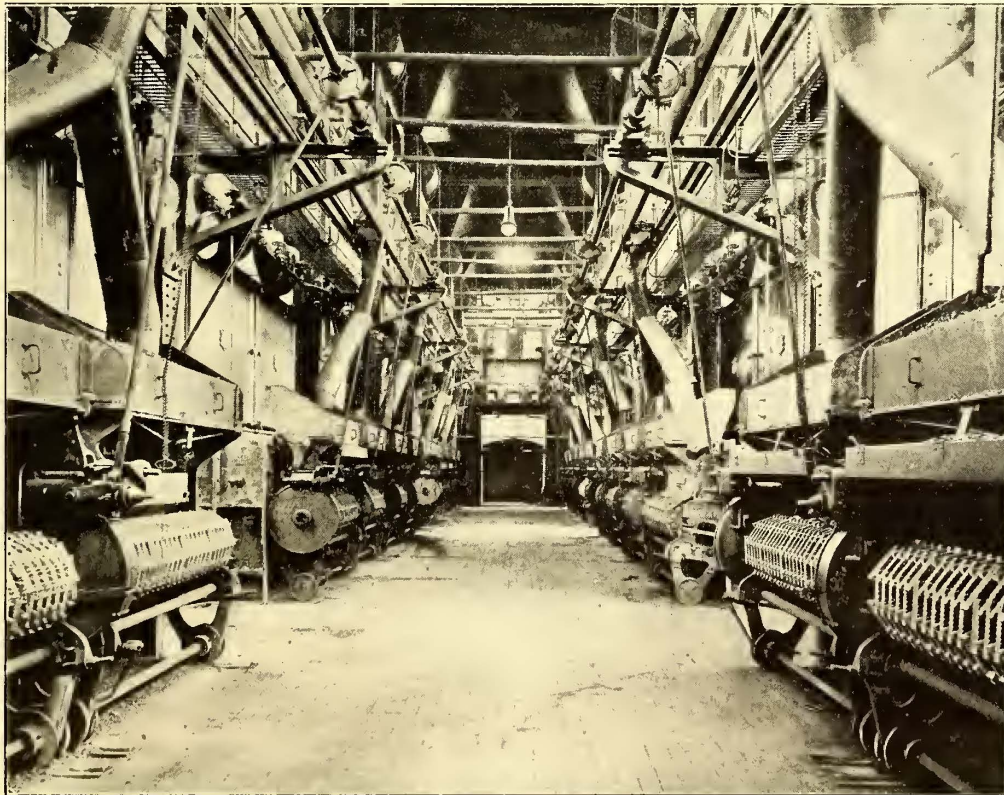
PARK ROYAL—GENERAL VIEW OF BOILER HOUSE FROM STOKING FLOOR
