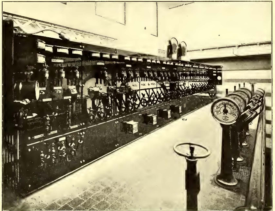
PARK ROYAL—NORTH MAIN CONTROL BOARD
