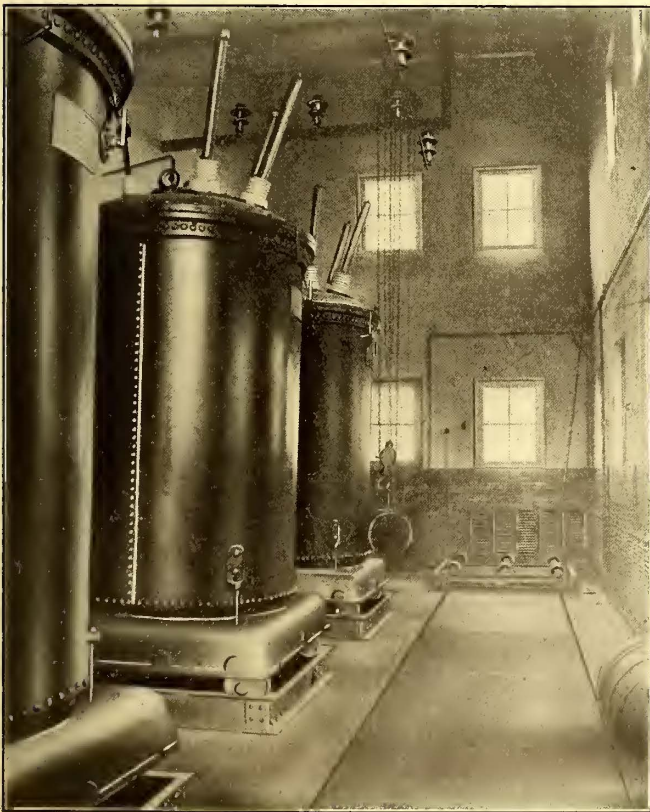
MAIN TRANSFORMER ROOM IN AVON SUB-STATION
