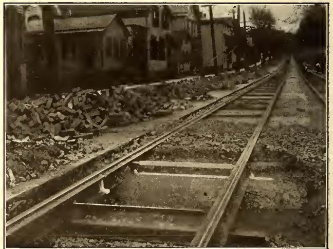
DETAIL OF TRACK CONSTRUCTION, SHOWING CONCRETE CONSTRUCTION WITH STEEL TIE EMBEDDED IN CONCRETE FOR PAVEMENT AND THERMIT JOINT
