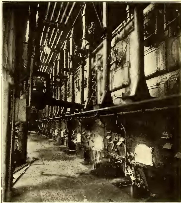
BOILER ROOM OF BARONNE STREET STATION.
