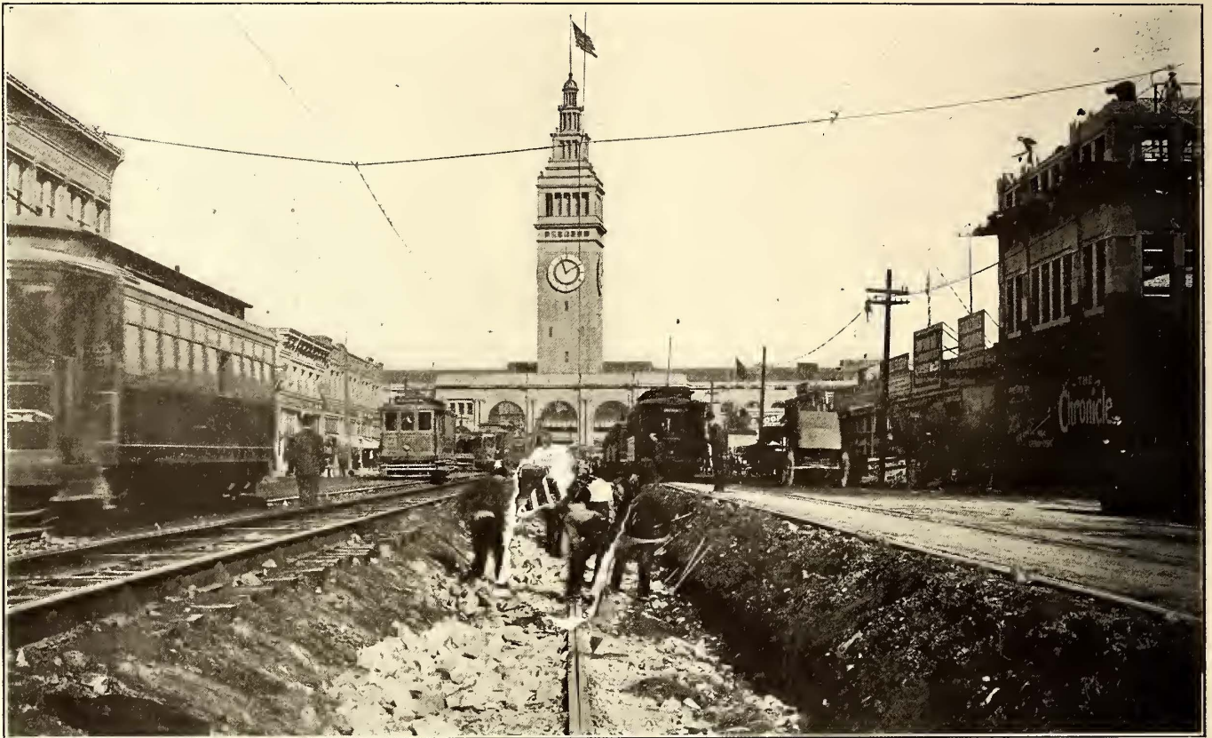
PULLING UP OLD CABLE RAILS, PREPARATORY TO FILLING IN AND RAISING ROADBED TO PERMANENT GRADE OF TRACKS AT SIDE
