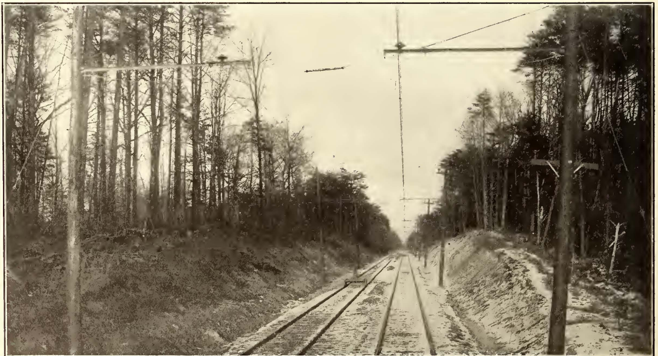
VIEW ON TANGENT, SHOWING OVERHEAD CONSTRUCTION AND METHOD OF TYING BRACKETS TOGETHER
