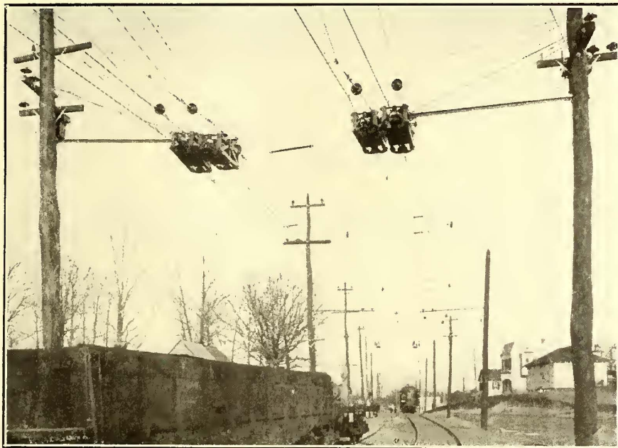
SECTION INSULATORS AT DISTRICT LINE IN WASHINGTON WHERE THE SINGLE-PHASE SYSTEM CONNECTS WITH THE DOUBLE TROLLEY DIRECT-CURRENT SYSTEM.
