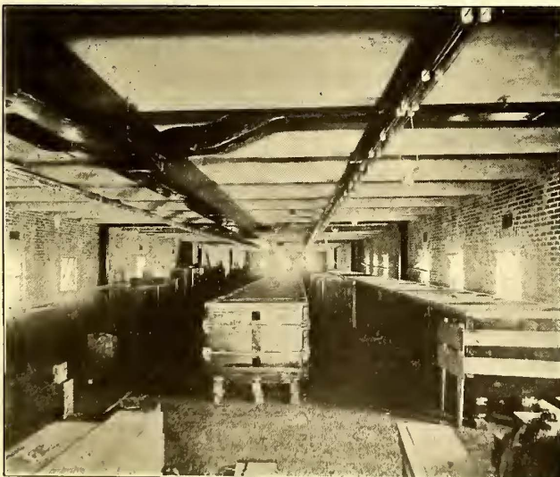
FIG. 2.—YONKERS BATTERY ROOM, SHOWING OVERHEAD DUCTS
