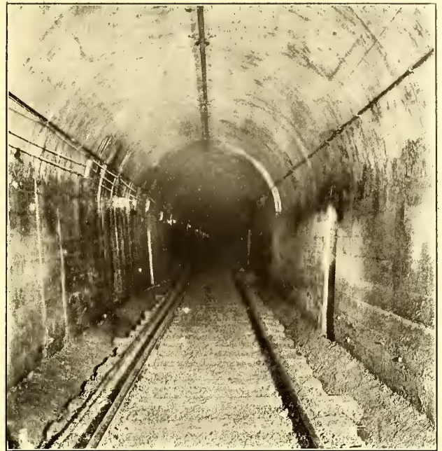
INTERIOR VIEW OF CONCRETE SECTION OF THE FORTY-SECOND STREET TUNNEL, SHOWING OVERHEAD CONTACTOR, ROADBED, ETC.
