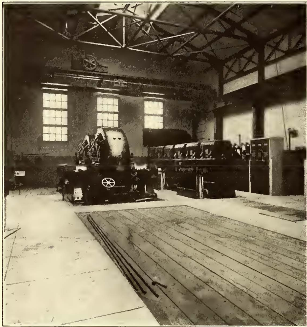
FIG. 19.—INTERIOR OF NEW PORTION OF NORTHERN SUBSTATION
