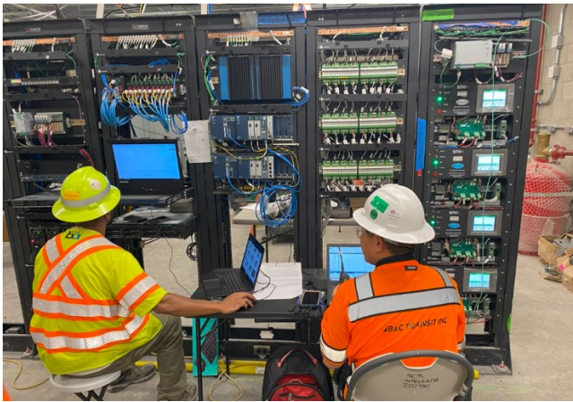
Wilshire/La Cienega Station SCADA Points Testing
