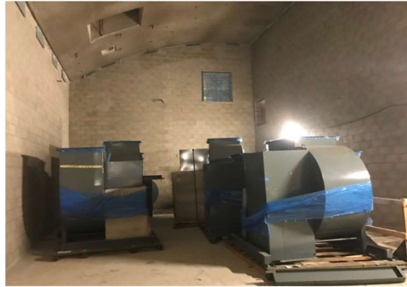
Westwood/UCLA Station: Equipment Staged in Ancillary Mechanical Room
