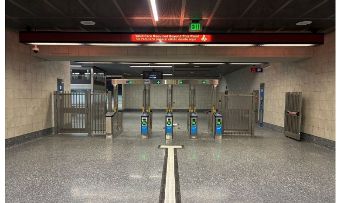
Wilshire/Fairfax Station Fare & Swing Gates
