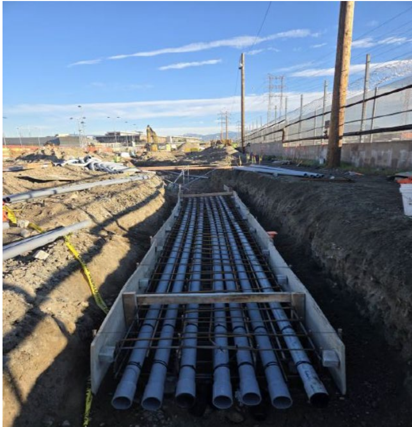
Installed contact rail ductbank at mainline track
