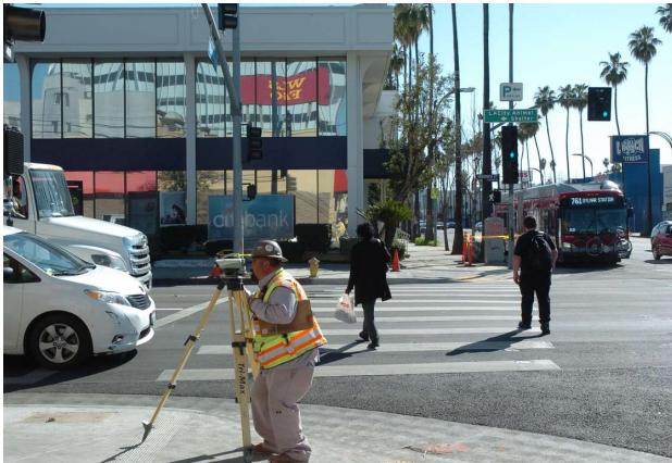
Preconstruction survey - Landmark surveyor establishing control point to the project site at the intersection of Van Nuys Blvd and Vanowen Street
