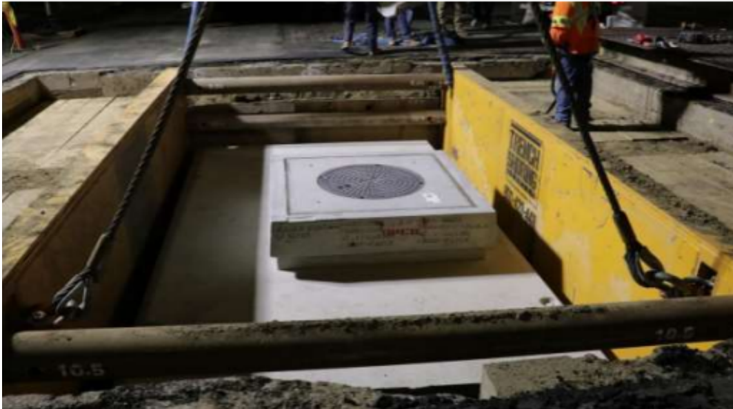
Vault 6834: Lower and upper vault are installed and aligned. Manhole cover is also placed.
