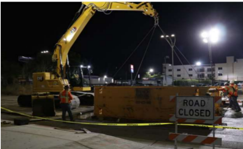
Vault 6834: Upper shoring box is place on top of the lower shoring box and locked.
