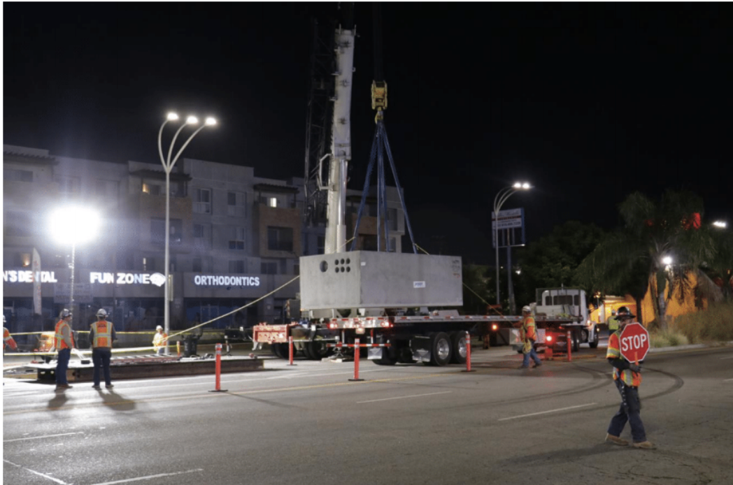
Vault 6834: Lower section of the vault is lifted by Good Guys crane while guide ropes on opposite sides give direction on placement.
