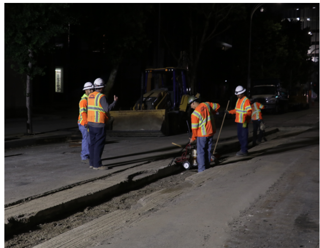
W.A. Rasic preparing the trench and applying Asphalt oil prior to arrival of Asphalt concrete.
