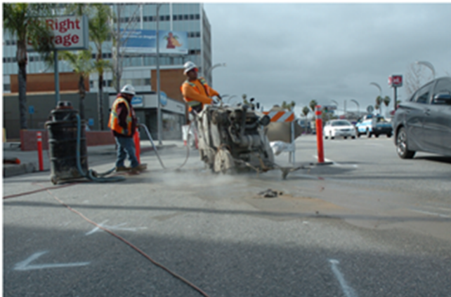
Utility Investigation: W. A. Rasic and Tom Grbavac crew slot trench asphalt to pothole on Van Nuys Blvd
