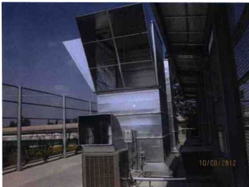
Guy cables on exhaust fans stacks.
