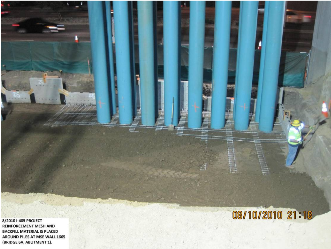
Reinforcement mesh and backfill material is placed around piles at MSE Wall 1665 (Bridge 6A, Abutment 1).
