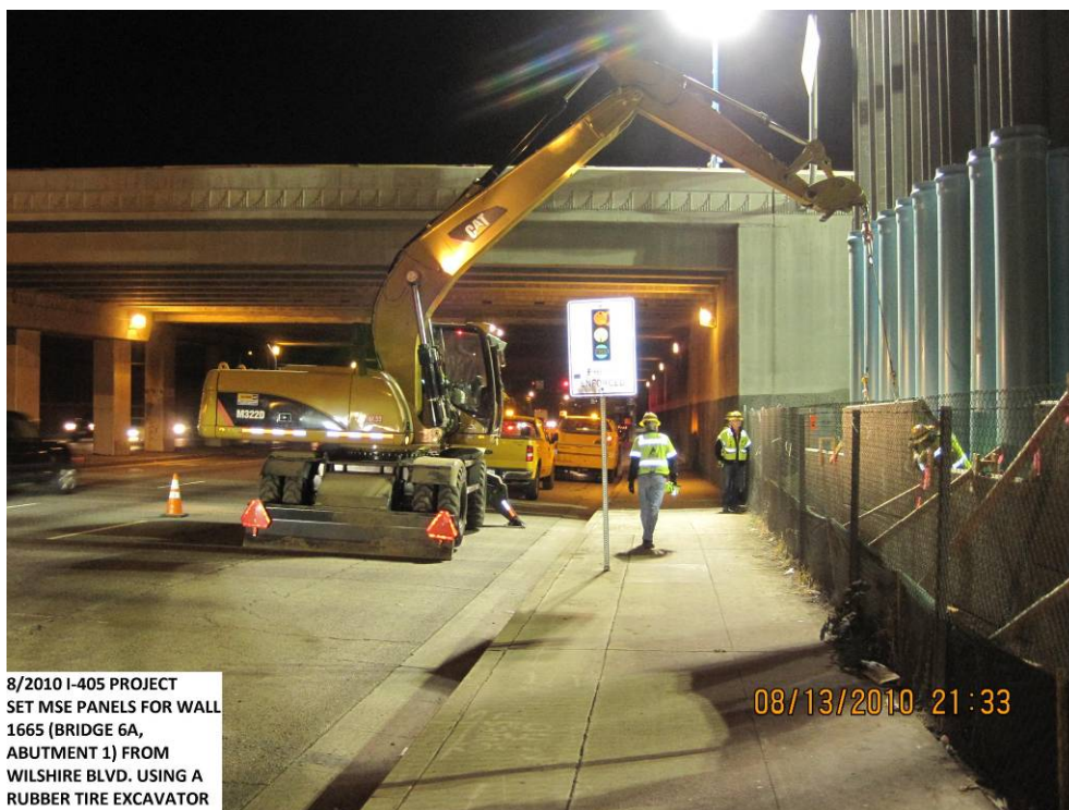
Set MSE panels for Wall 1665 (Bridge 6A, Abutment 1) from Wilshire Blvd. using a rubber tire excavator.
