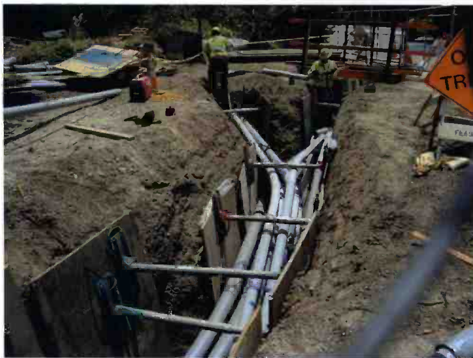
Ductbank on Sepulveda Blvd. at Homedale.
