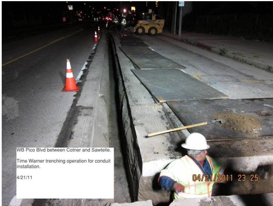
Time Warner trenching operation for conduit installation WB Pico Blvd. between Cotner and Sawtelle.
