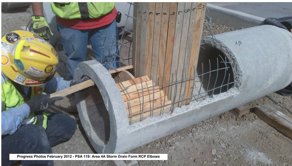
PSA 119: Area 4A storm drain form RCP elbows.
