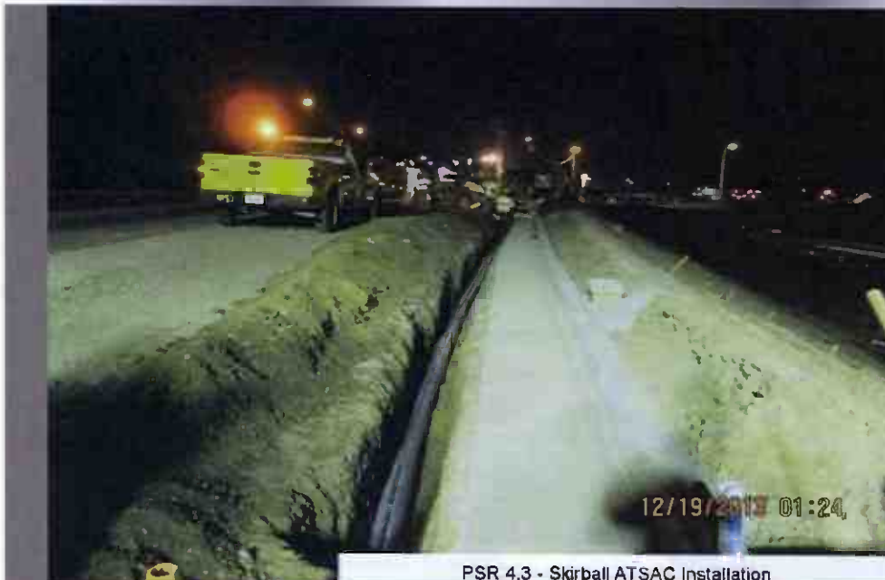
PSR 4.3 - Skirball ATSAC Installation
