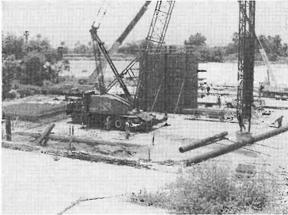
Contract C0676 pile driving and pier construction activities at Los Angeles River Bridge site.
