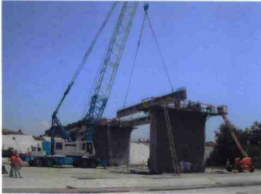
Contract C0676 Los Angeles River Bridge. Contractor lifting prestressed precast concrete girders onto bridge piers.
