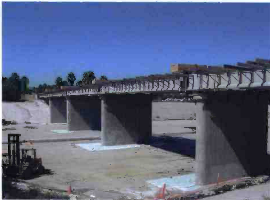
Contract C0676 Los Angeles River Bridge. Contractor completed lifting the twenty girders onto bridge piers.
