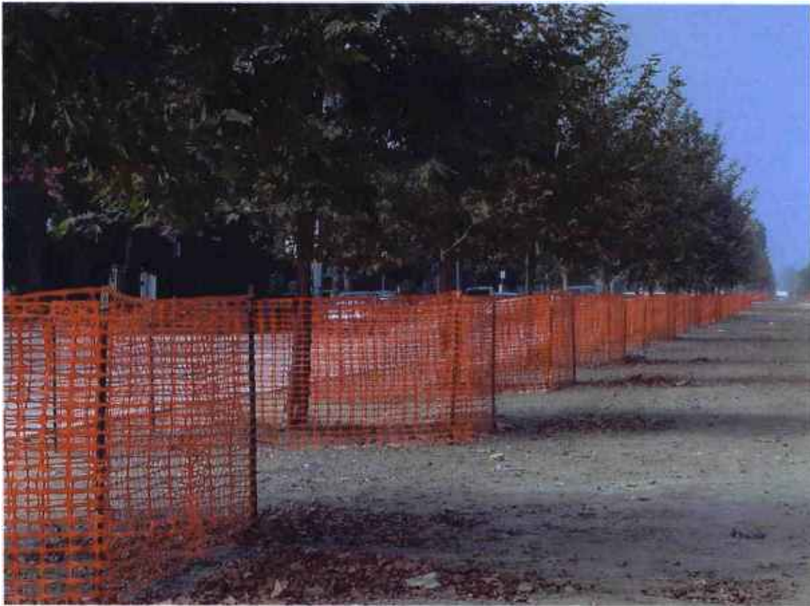
Contract C0675 Design/Build Contractor has placed tree protection fencing along east end of busway along Chandler Boulevard.
