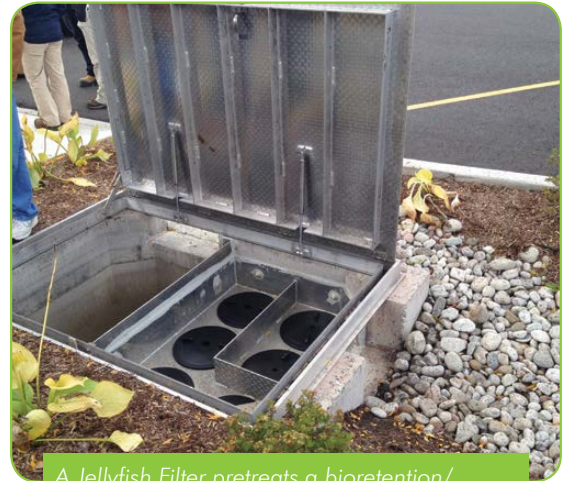
A Jellyfish Filter pretreats a bioretention/bioswale system at a commercial site in Ontario, Canada.
