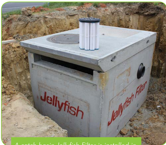
A catch basin Jellyfish Filter is installed in a commercial development in Virginia.
