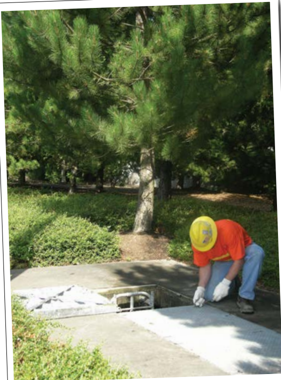
StormFilter structures can be accessed without confined space for inspection.
